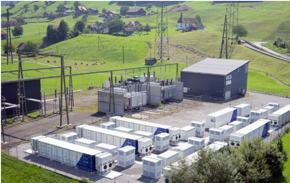
The battery storage unit in central Switzerland has a power of 20 MW.
